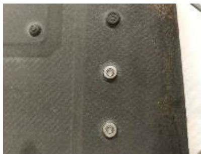
Fig 3- Installed Blind Rivets with Coating Removed
